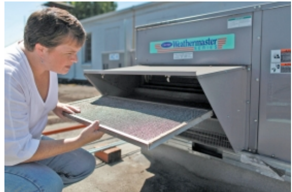
JAIME VALDEZ / PAMPLIN MEDIA GROUP Tammy Stempel, Gladstone planning commissioner, checks air filter on City Hall rooftop to improve heating and ventilating system's energy efficiency.
